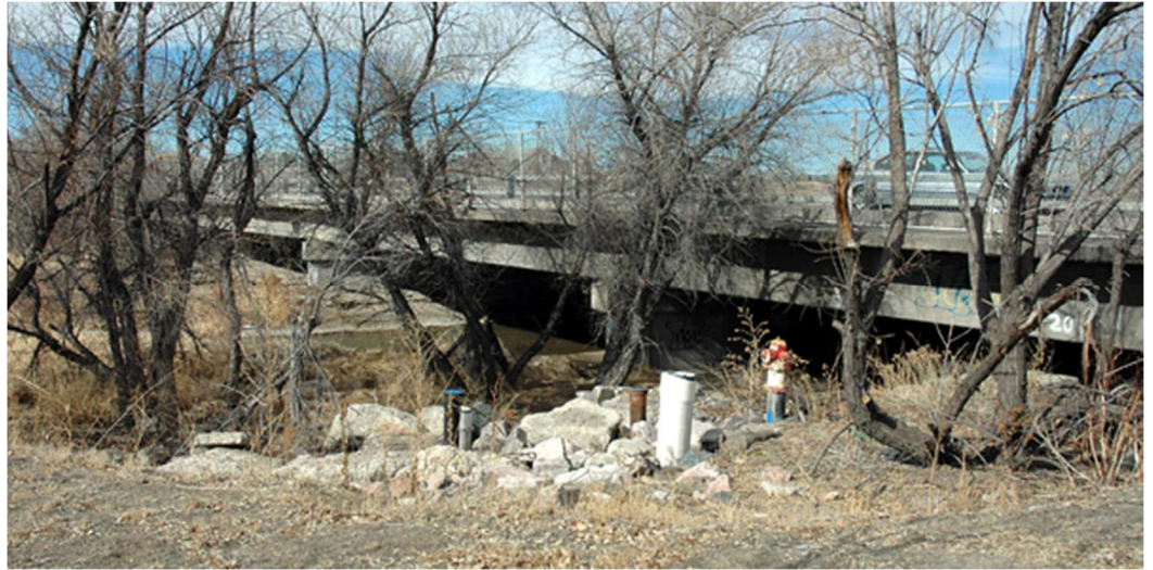
Here's the Arapahoe Road Bridge over Cherry Creek on the south side where a low-water pedestrian bridge is in the works as a step to close the trail gap.
