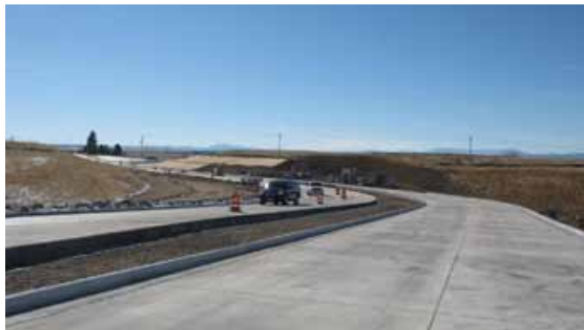
The new ramp from northbound Parker Road to eastbound and westbound Arapahoe Road is open.
